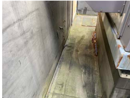
Image 2 – Monitor Well EPDM roof and walls.
